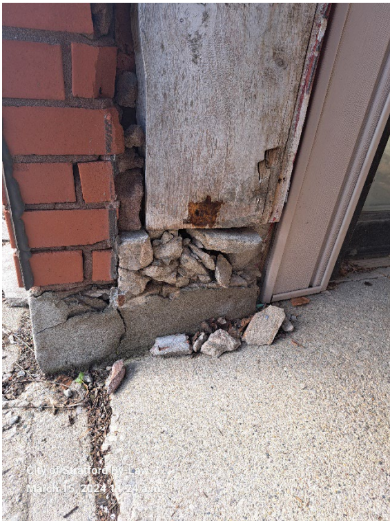
- Deteriorated/missing concrete/brick at the front entrance.
