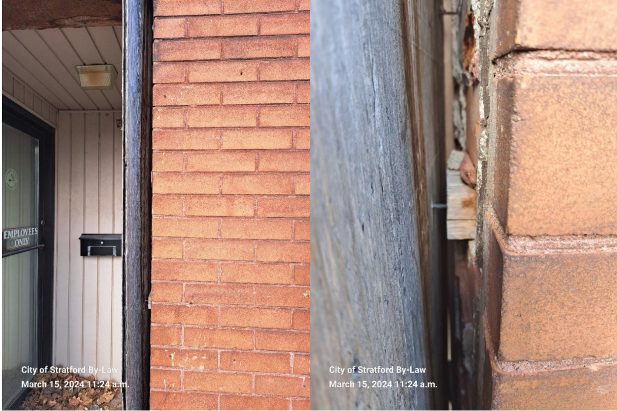
- Deteriorated wood around front entrance.
