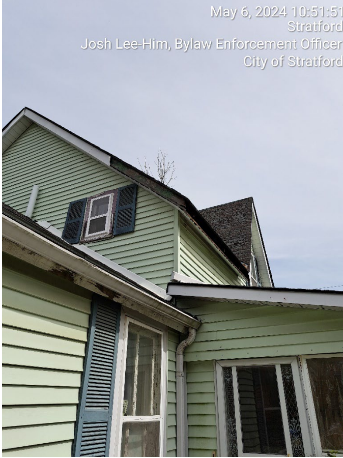
Roof in disrepair and further damage to soffit and fascia.
