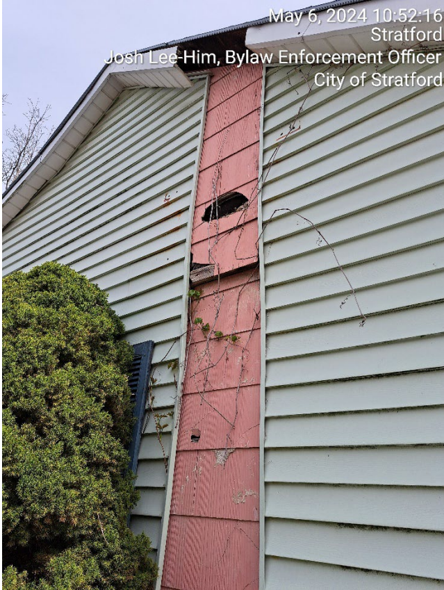
Hole in the side of the exterior wall, as well as soffit/fascia in disrepair.
