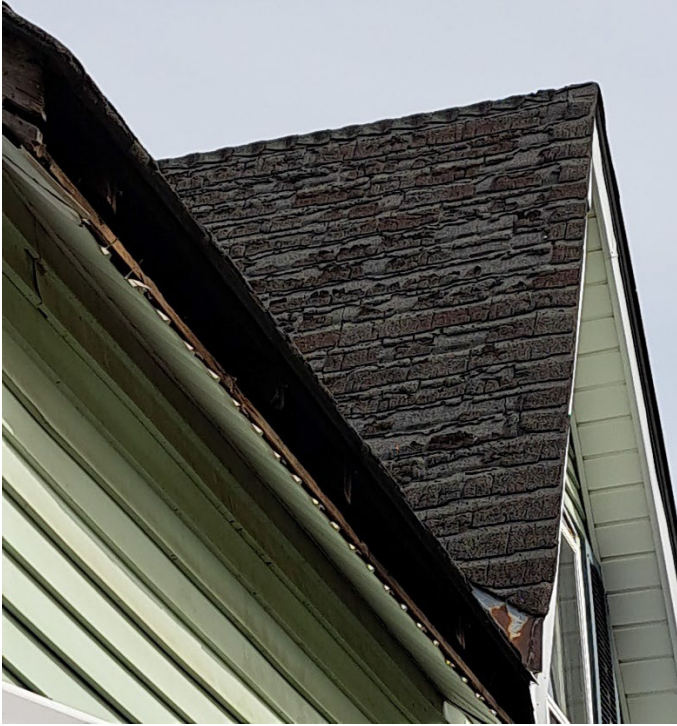
Roof, soffit and fascia in disrepair.
