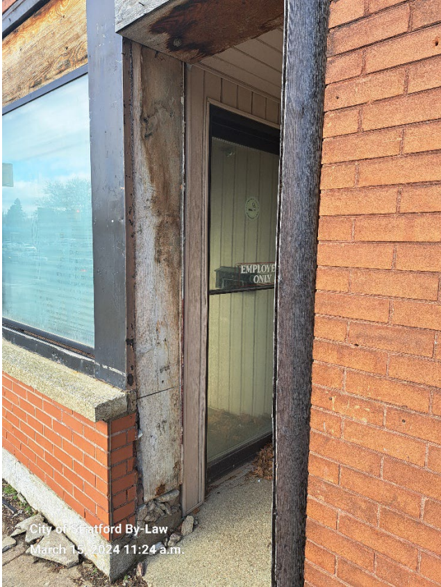
- Deteriorated plywood around front entrance.
