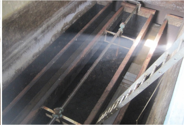
Interior of a filter
