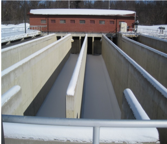
Chlorine Contact Chamber
