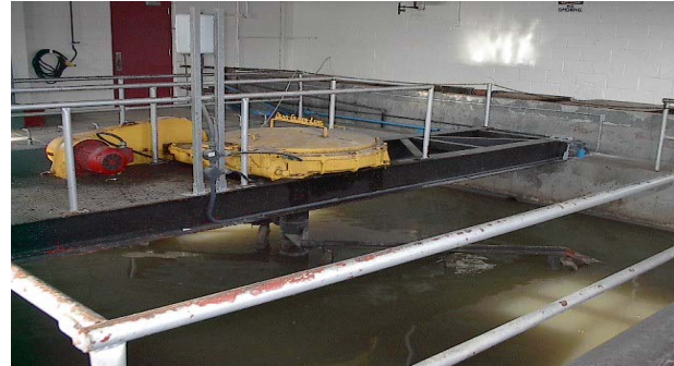
Grit removal system
